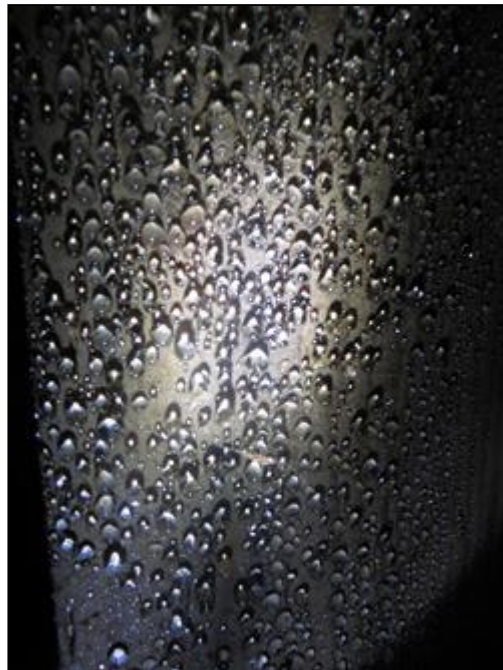
Water Accumulation From Condensation At Beams
