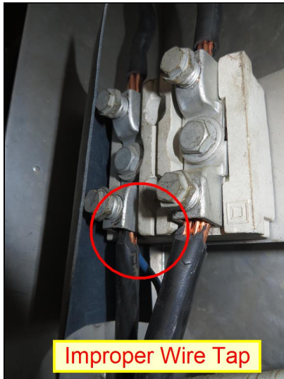
Cant Verify Protection of Circuit
