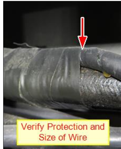
Improper Wire Tap
